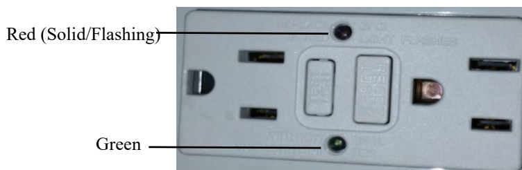
Figure 3. NEMA 5-15 Receptacle Lights
